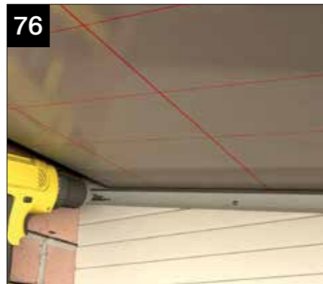
76 For the roof panel adjacent to the firring, after fitting the 90mm insulation, screw fit CHA405/1 channel where the 90mm insulation converges with the inside face of the firring using CHAA006 fixings. This serves to carry the edge of the 25mm insulation and offers a surface to screw the plasterboard to. The channel should span front to back.
