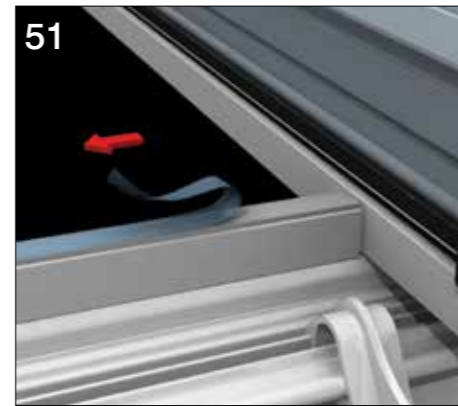
Tease the 'tail' of the glazing support trim tape free (ready to be pulled away when the sealed unit is finally in position). This will need to be pulled inside the roof at the front as access will not be possible once panels are fitted. The rear film maybe easier to access externally.
