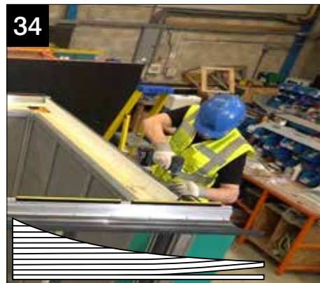
Separate the firing frame connector from the firings and position the frame connector onto the cill and secure down into the walls/frames. Fixing FRFC008-100 has been supplied for the fixing into the walled sides. Suitable fixings into frames are to be sourced separately.
