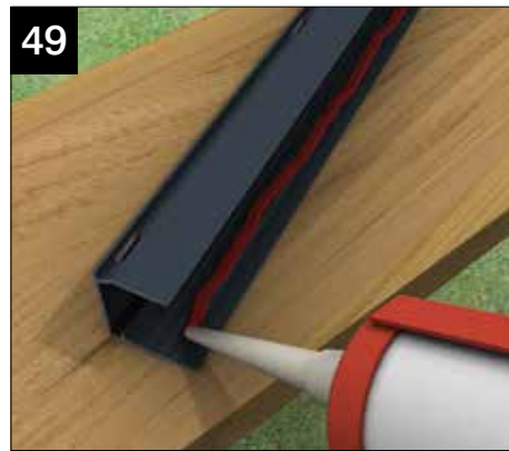
Take the coated profile and protect its surface. Apply a bead of relevant sealant (MS polymer on self cleaning glass). Slide into position on panel and/or glass, wipe clean any sealant from surface.
