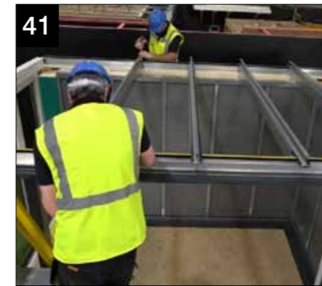
Lower roofing bars onto eaves beams locating bolts, between glazing supports and secure in place with nuts.
