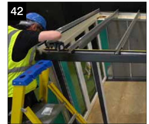
Offer up the long cornice mid section into position along the front of the structure and secure using fixings provided (CHA007) at 400mm centres.
