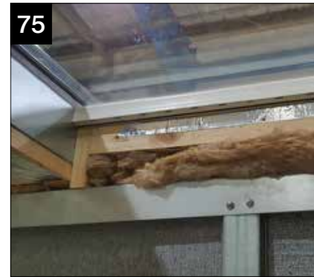
75 The frame, previously constructed, should sit flush with the walls then fix into the bolstered element of the roof bars. Once fixed fill the void below the panel with mineral wool.
