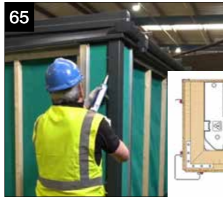
65 Run a continuous bead of sealant along the corner claddings and the cladding clips as shown.
