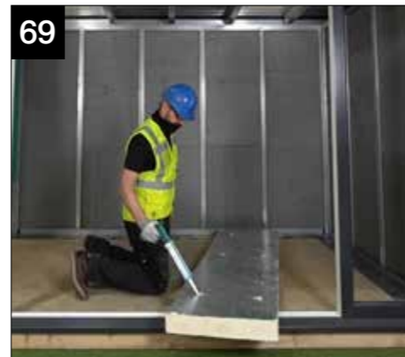
69 Now moving onto the installation of the insulation. Take the 90mm insulation board - each part is numbered/lettered to identify where it goes (label always to the inside of the structure). Spot the board with sealant. It may be necessary to cut the insulation for ease of fitting, seal these joints using foil tape (LVFT045). Fitters Tip: Cut insulation in half for ease of fitting.
