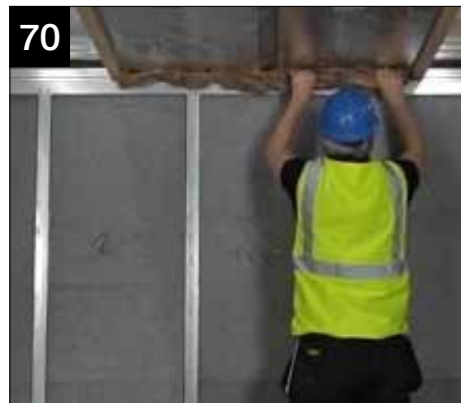
70 Use mineral wool to close any gaps between 90mm insulation and eaves beam and along the top of the walls.
