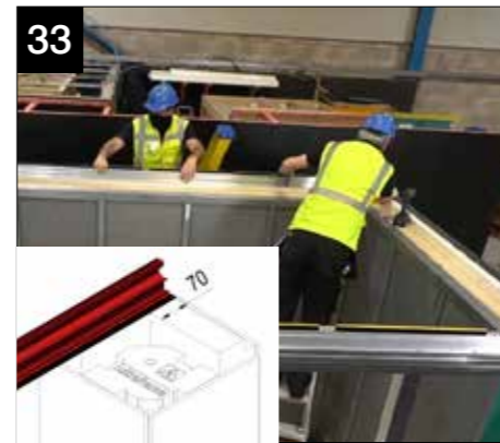
Locate the rear eaves beam onto the cill aligning to the inside upstand and fix down through the cill into the top tray timber using fixing NRDS070.
