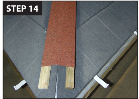
Place the Ridge cap over the battens to set the width of the battens at the bottom, mark each side of the batten.
