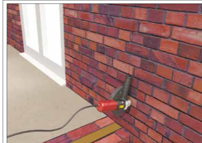
When using abutment columns, a vertical DPC is required between the column and host wall.
